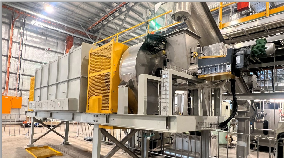
HPA dryer installed into Stage 1
