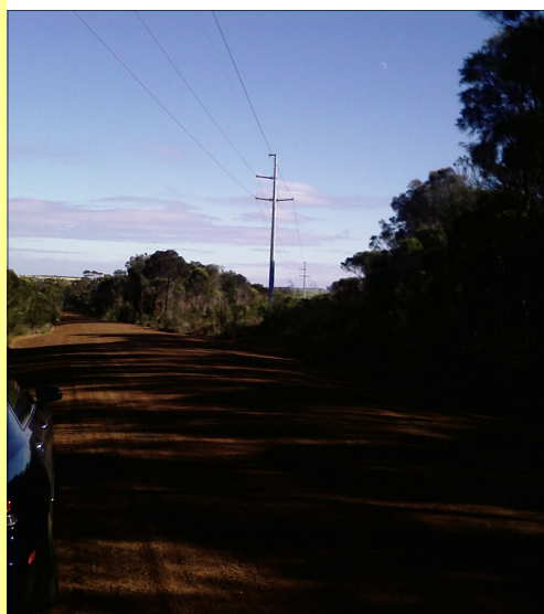
66 kv powerlines near Red Hill at Katanning
