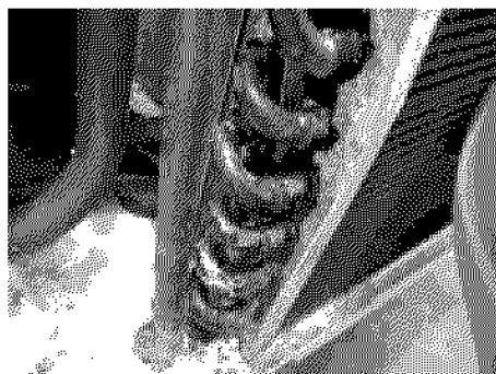
Example of severity of coil corrosion on rooftop HVAC unit
