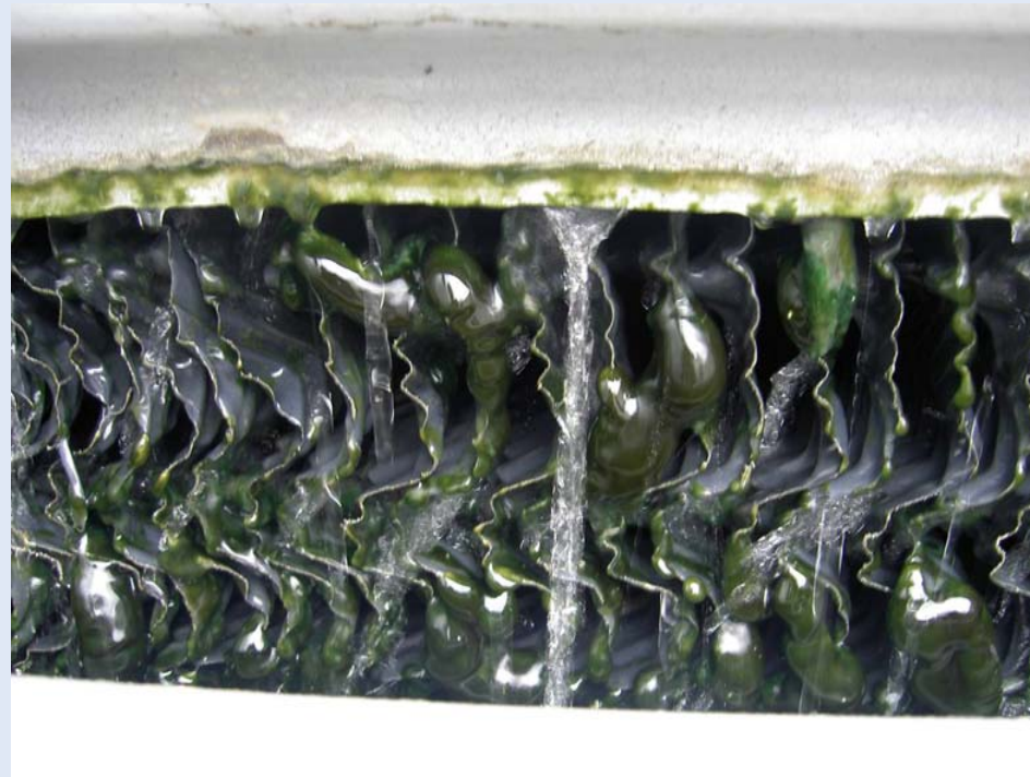
Biofilm in cooling tower
