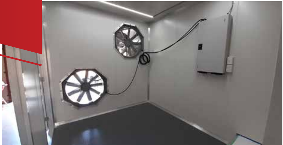
Inside of the prototype modular data centre, note- not-to-scale
