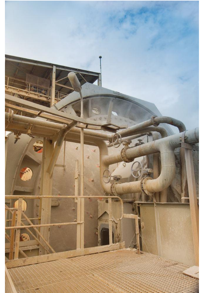
Single stage 3.5 MW SAG Mill.
