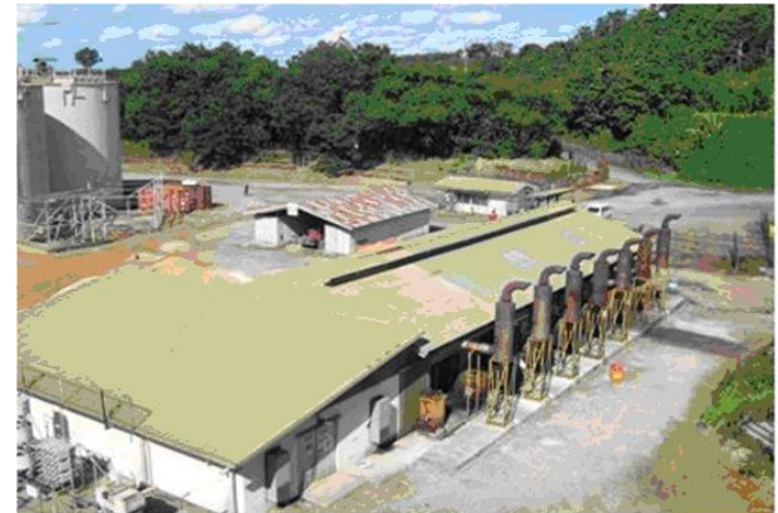
4.7 MW Diesel Power Station
