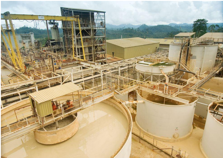
Mt Muro Leaching Circuit
