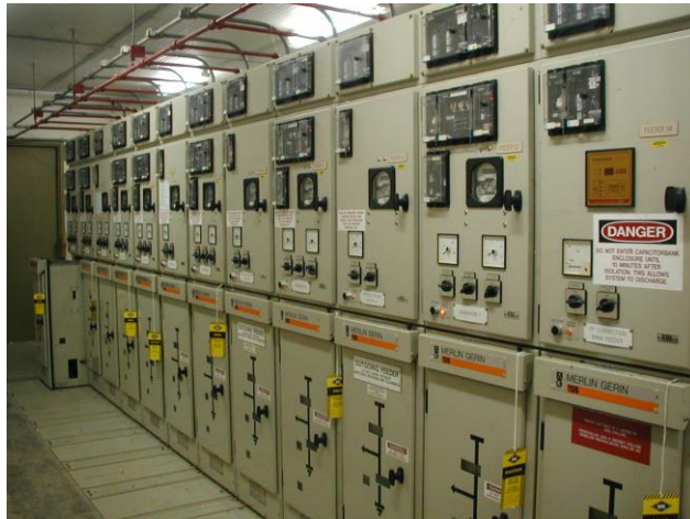
Network distribution and control
