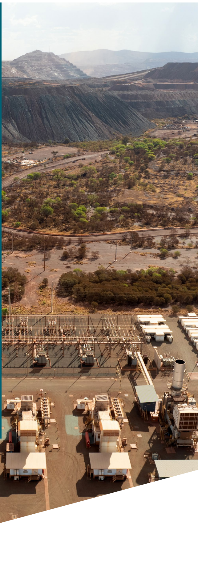
Newman Power Station, WA
