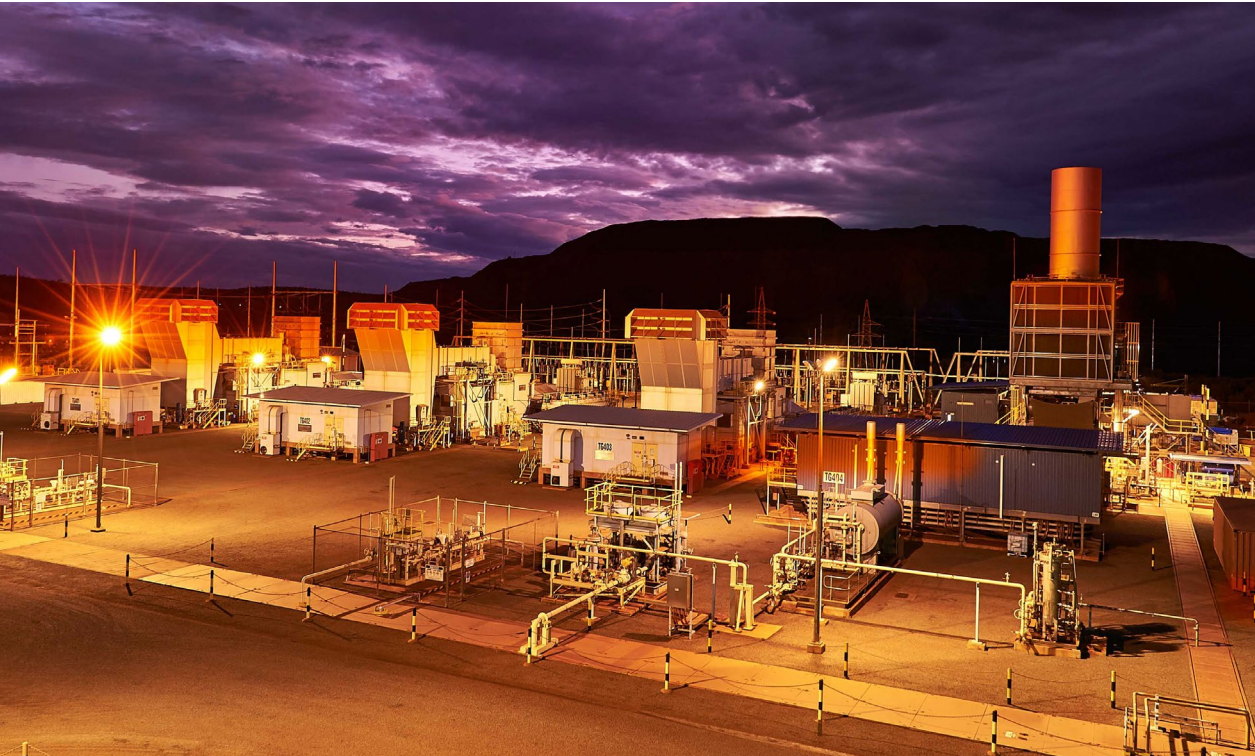
▲ Newman Power Station, WA
