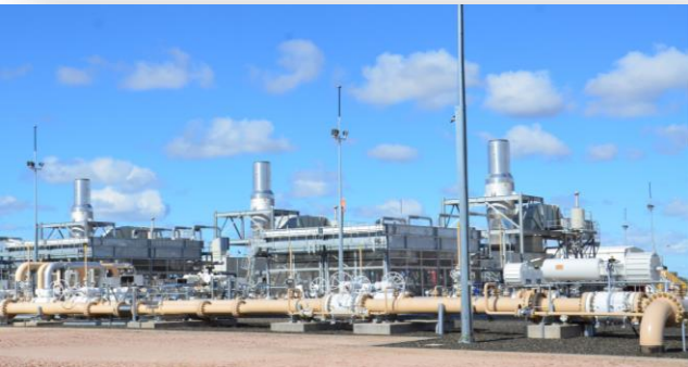
Wallumbilla Compressor Station
