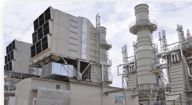
Diamantina Power Station in Queensland
