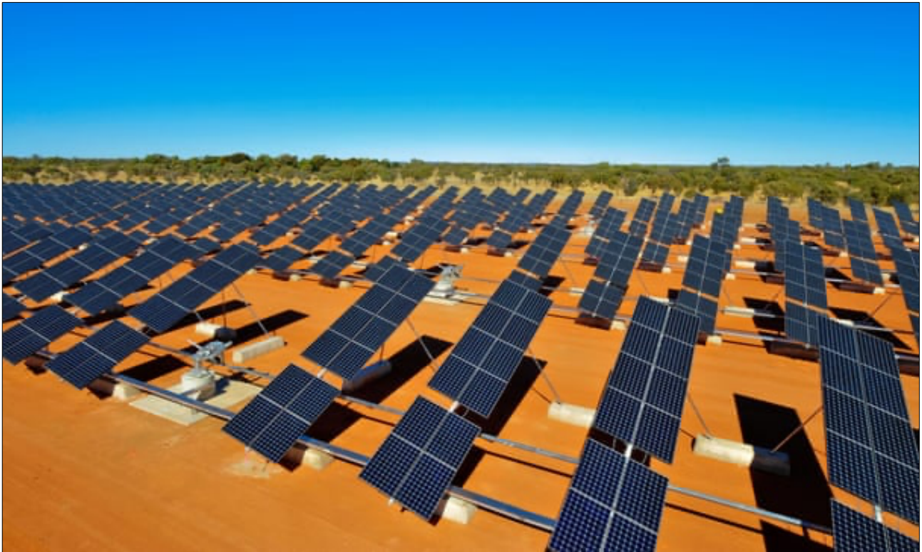
Figure 8 A large solar array will be developed
