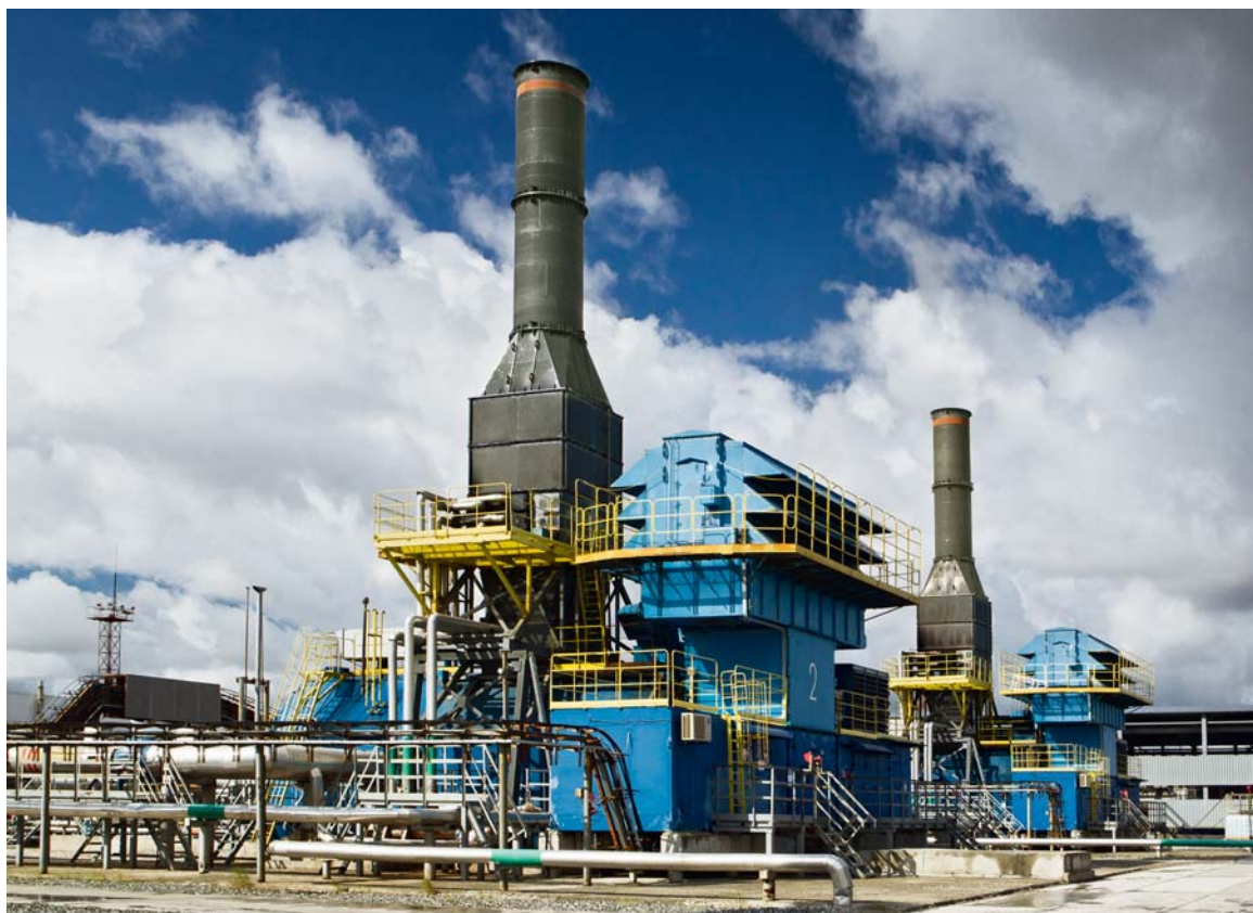
COMPRESSOR BOOSTER STATION AT THE EAST-TARKOSALINSKOYE FIELD
