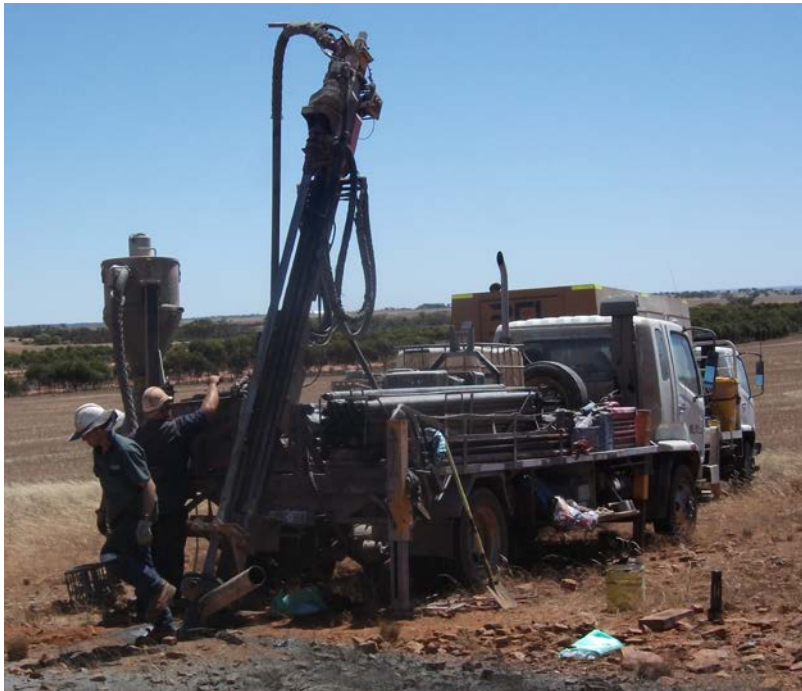
Figure 1. Photo of the RC drill rig used for the February drilling program at Bencubbin, Western Australia.
