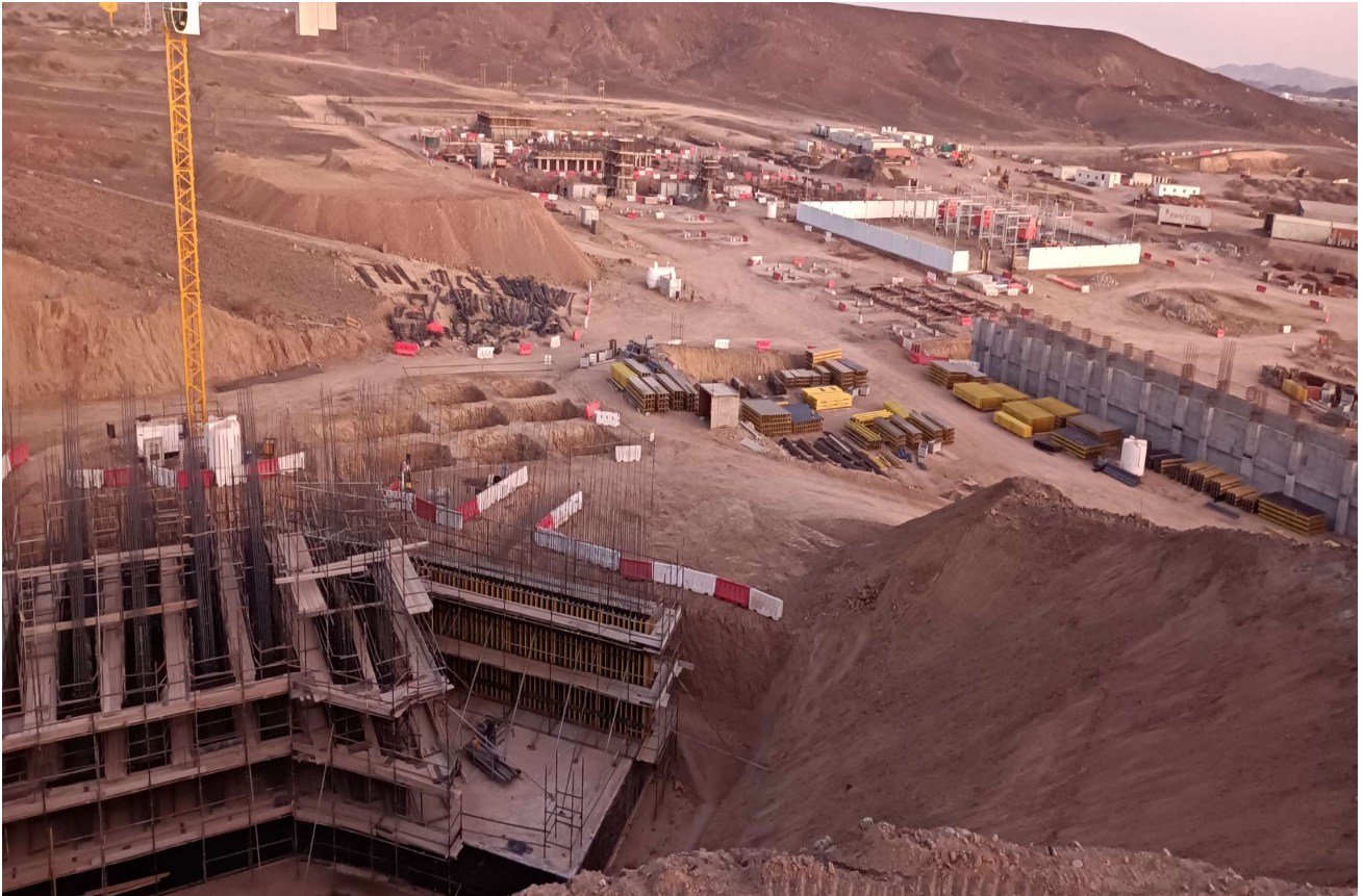
Primary crusher area close up
