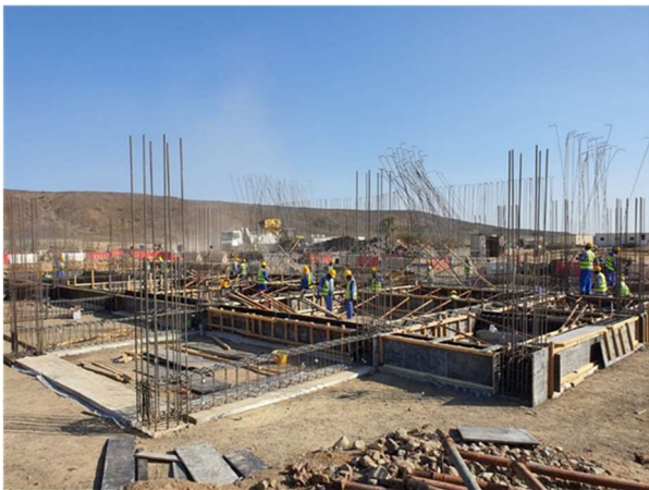
Grinding area electrical building
