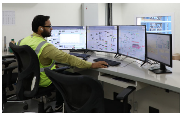
Plant control room
