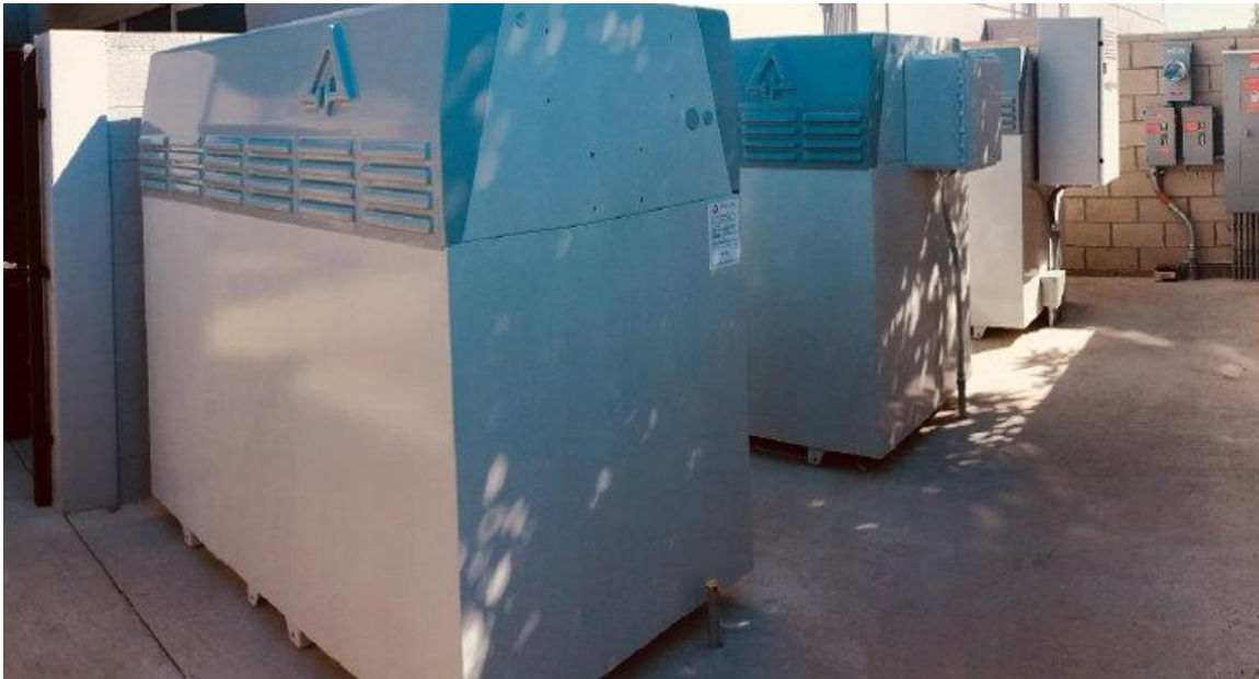
Figure 10 – Invinity Energy Systems VRFBs
