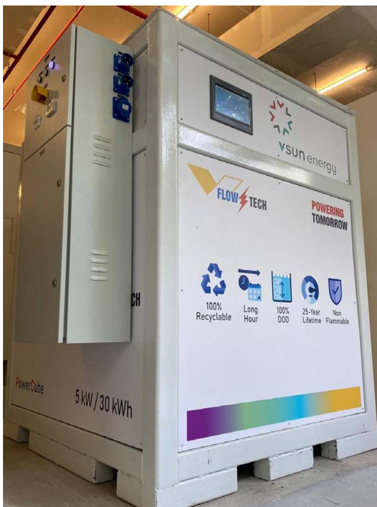
Figure 6 A 5kW/30kWh V-Flow VRFB
