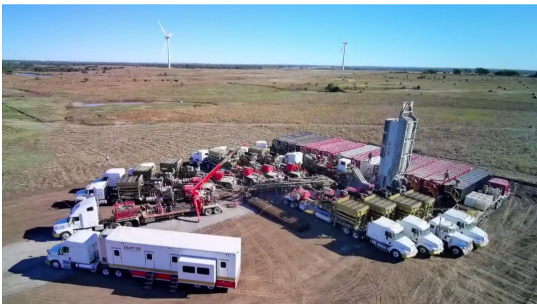
Figure 1: Photo of today's operations at the Charlie #1 Well
