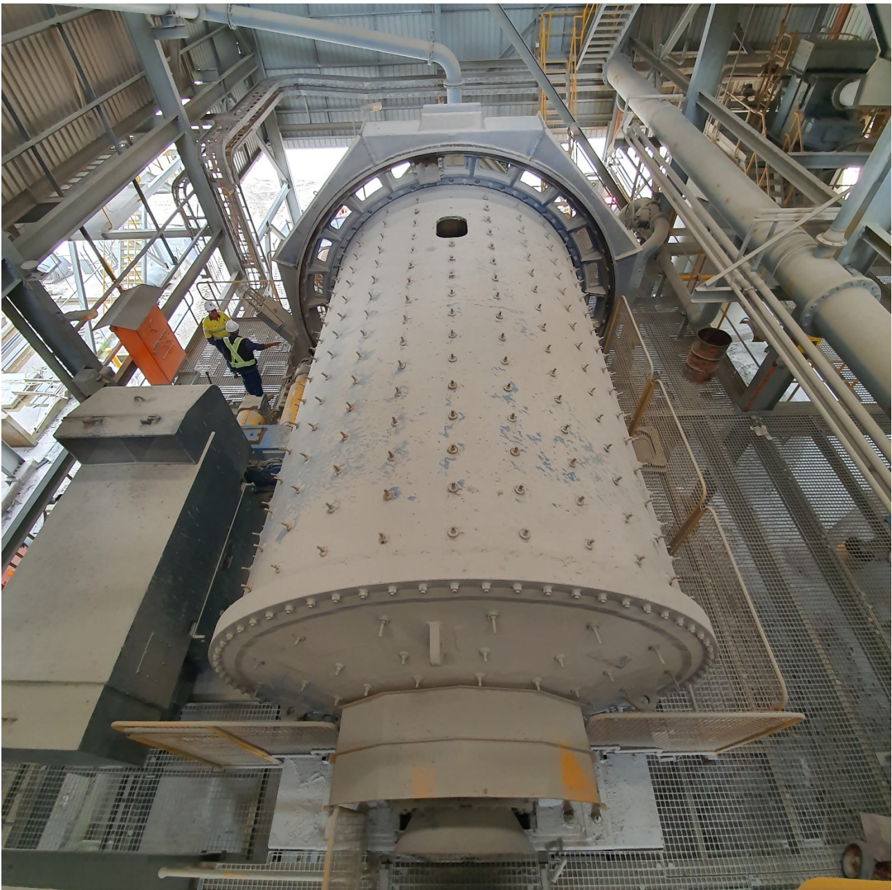
Figure 2: 1.85MW Outokumpu ball mill
