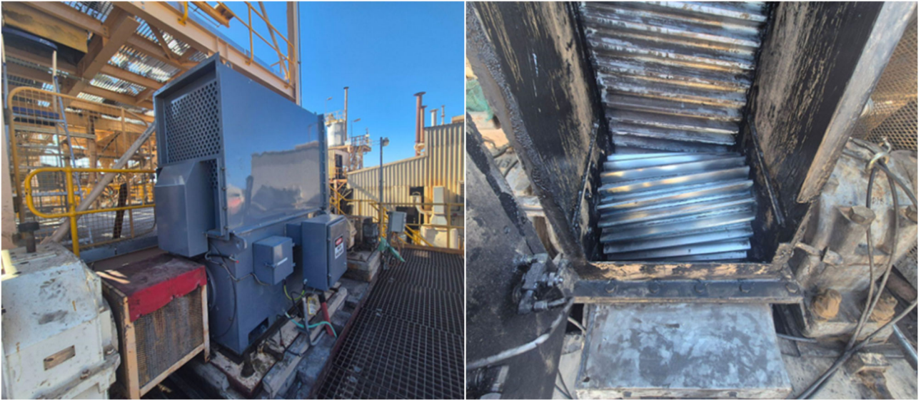
Figure 3: The refurbished ball mill motor has been installed and pinion gear installed and fully aligned.
