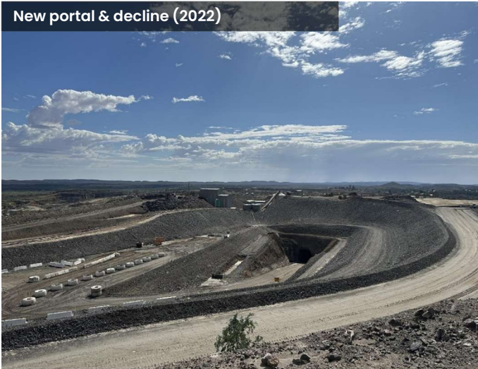
750,000tpa capacity processing facility
