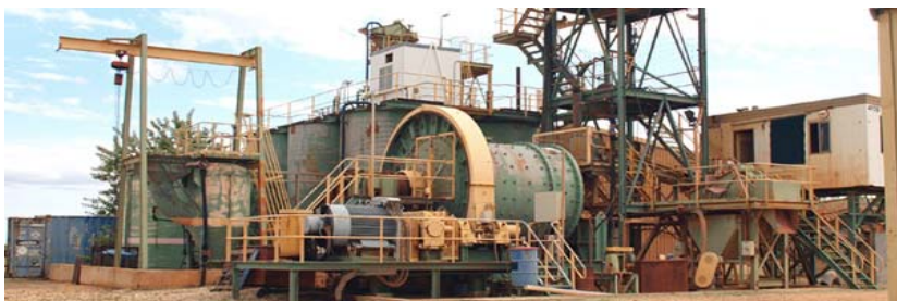
Existing Processing plant
