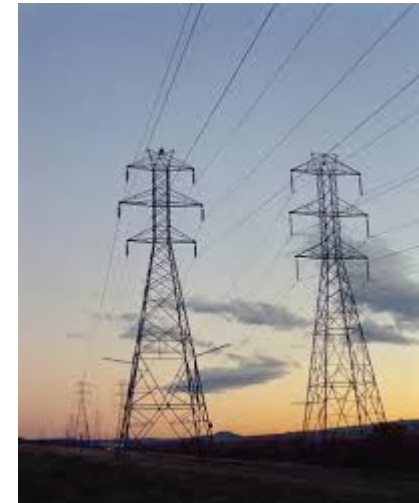
High voltage power through permits
