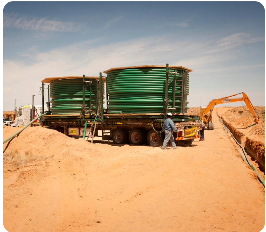
Pipeline capital cost and laying time reduced through use of Fibrespar flexible pipeline
