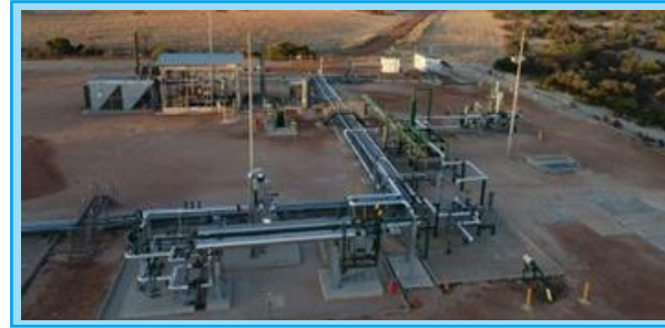
Xyris Gas Plant
