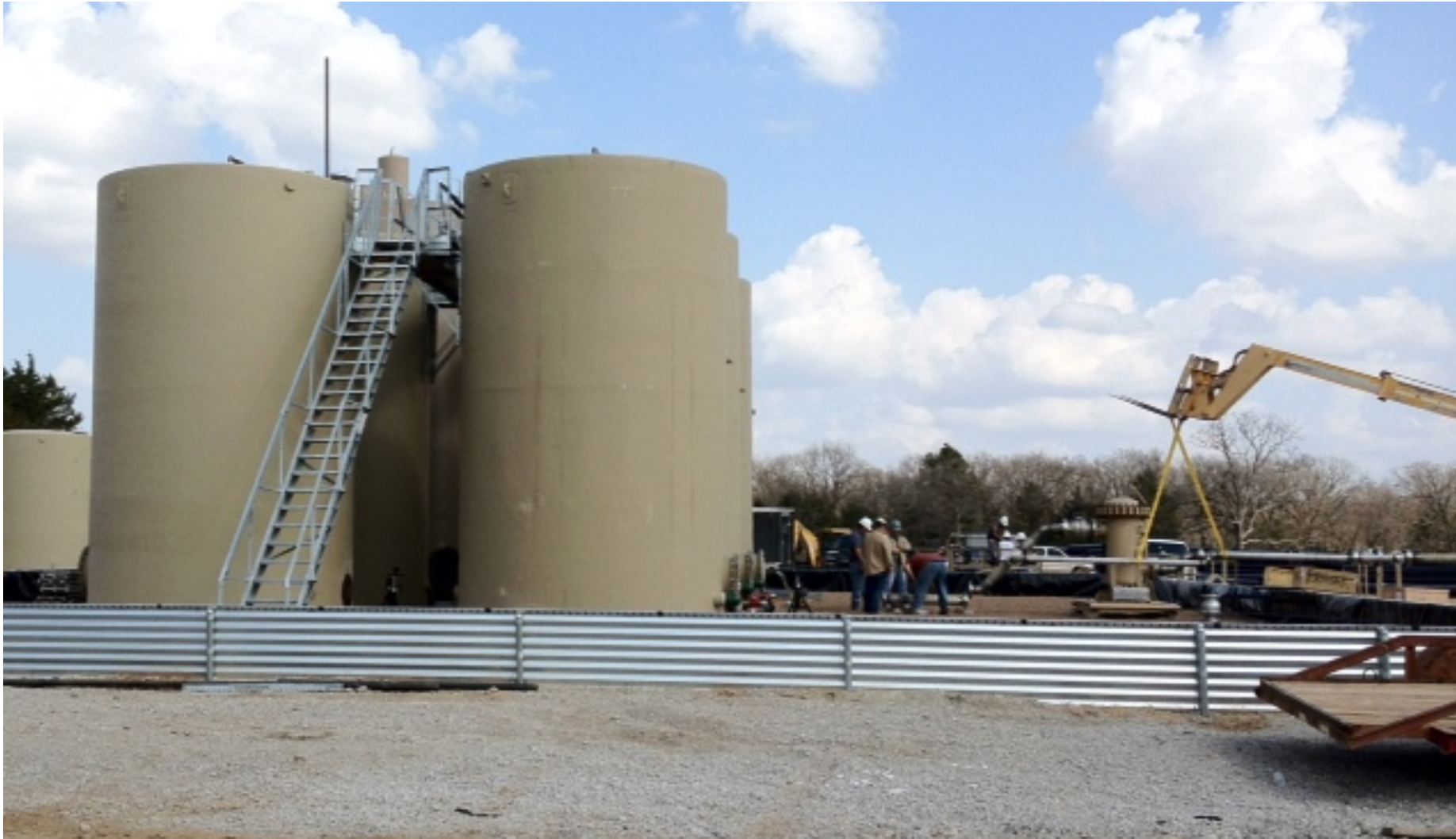
Central Delivery Point & Produced Water Disposal Facilities, Noble County
