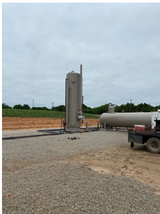
Figure 3. Surface production facilities
