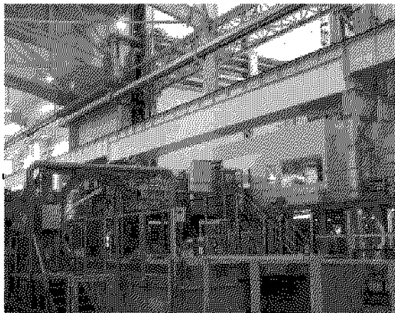
金属镀层生产线/Metallic Coating Line
