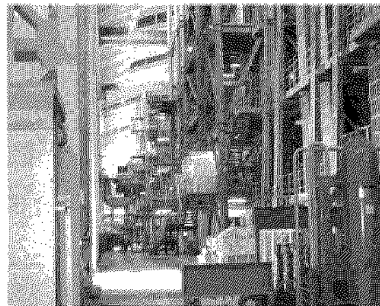
金属镀层生产线/Metallic Coating Line
