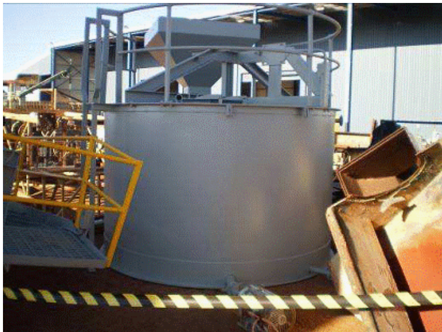
Mixing Tank with band and Surface Treatment
