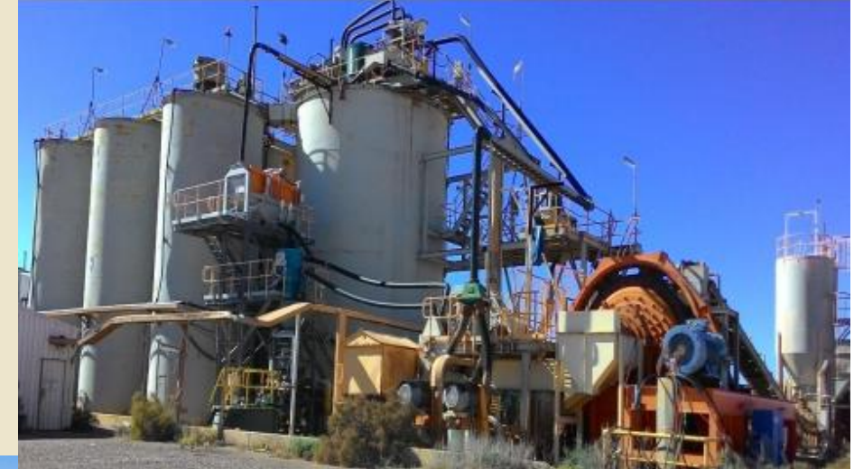
Processing Plant & Infrastructure in Laverton
