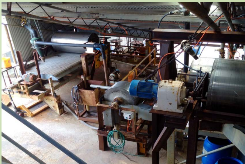
Re-start Processing plant (grinding, gravity, flotation)
