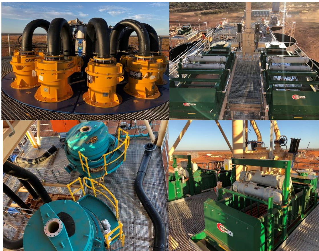
Process plant equipment installed
