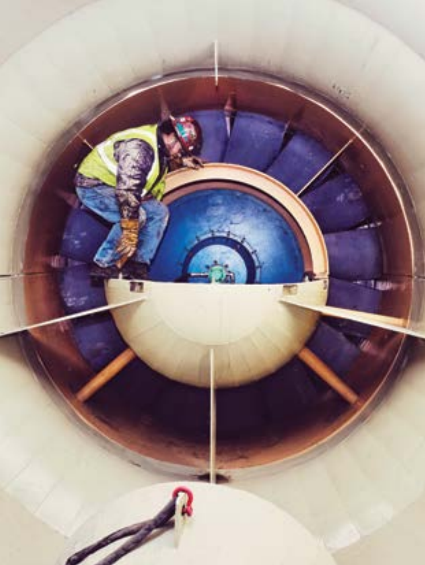
Above Ventilation maintenance at Buchanan
