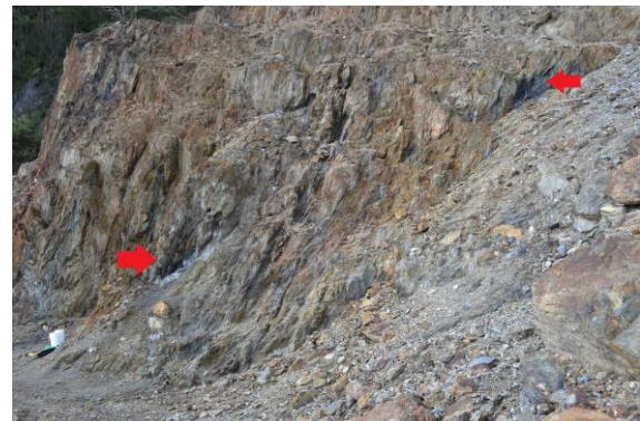
Above: At the centre of the Gibson mine a wide exposure (~15m width) of zinc, lead, copper mineralisation is observed. The bucket to the left of the picture is at the opening of the adit
