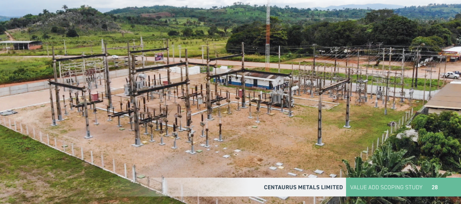
Figure 19 - 138kV National Grid connection at Tucumã
