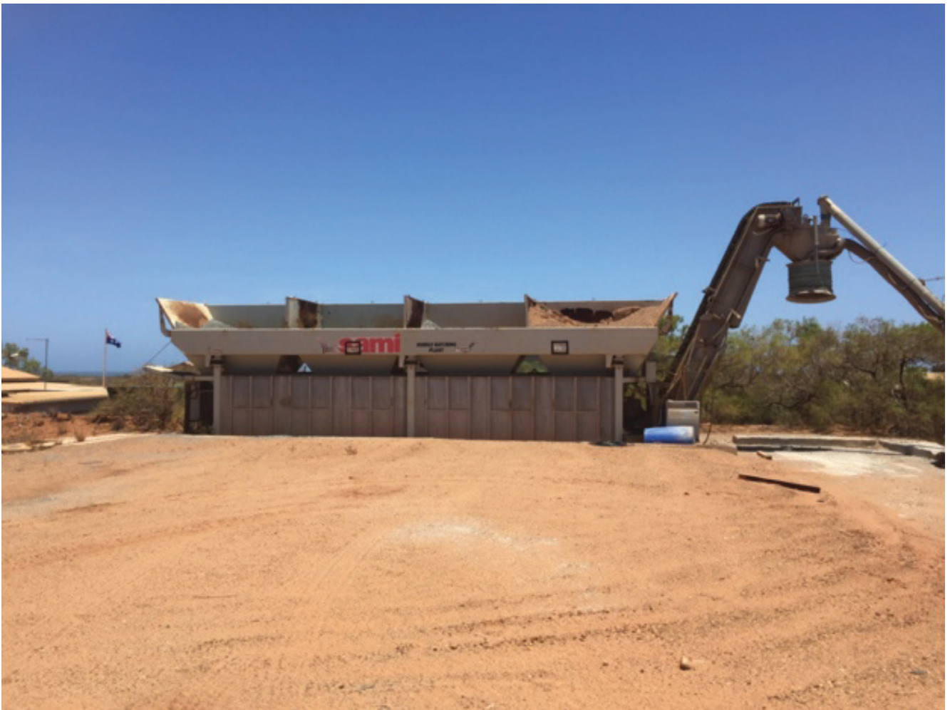
Figure 8: T4 Sami Mobile Concrete Batching Plant, Lot 697 Cornish Way, Onslow
