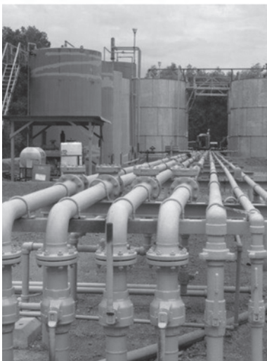
Tank Battery and Flow lines
