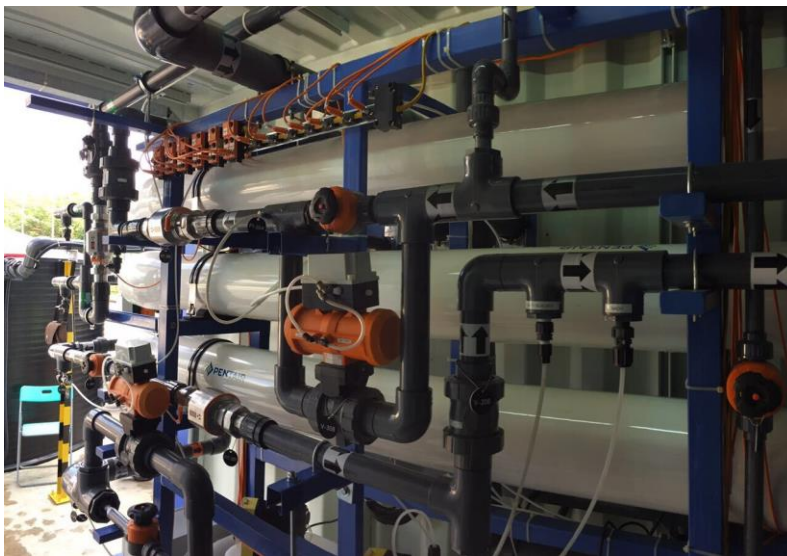
Interior of containerized waste water treatment plant built by De.mem at a customer site
