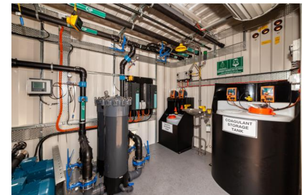
IMAGE 4: Chemical dosing system
