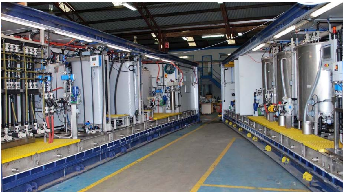
Figure 1 – PhosEnergy Process Demonstration Plant
