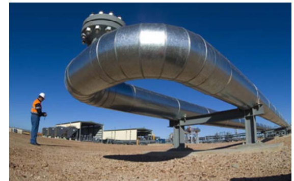
Arrow Energy gas processing facility
