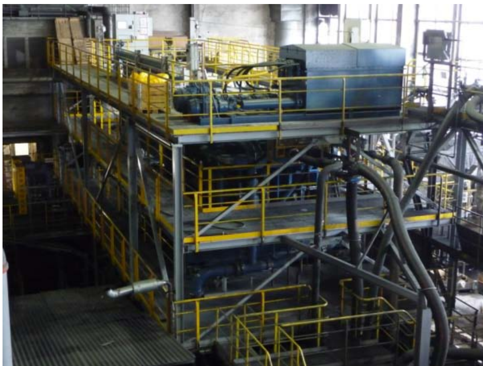
Figure 4 - completed pressure filter
