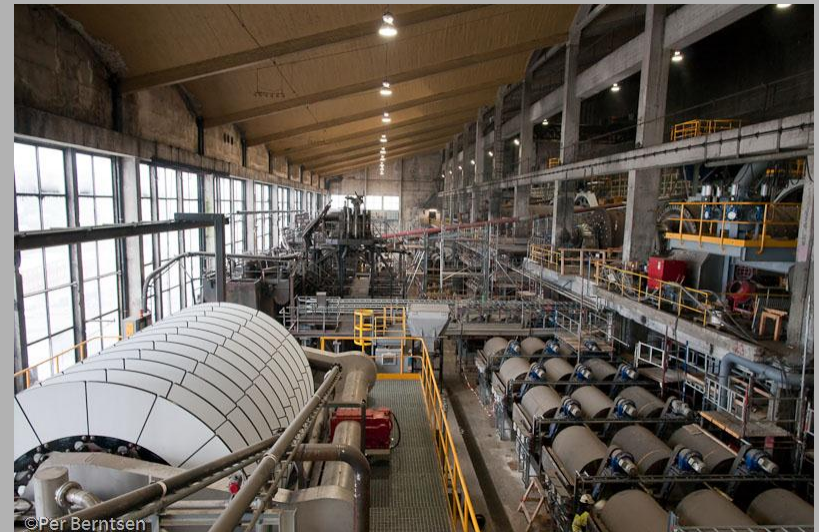
Refurbished magnetic separators, old and new filters
