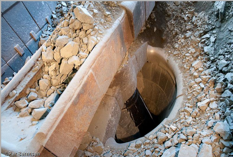
Refurbished primary crushers
