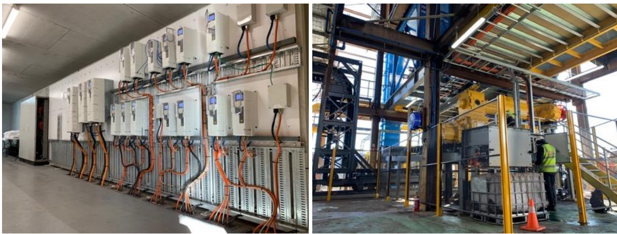
Photos (above): Programming of primary process control systems.
