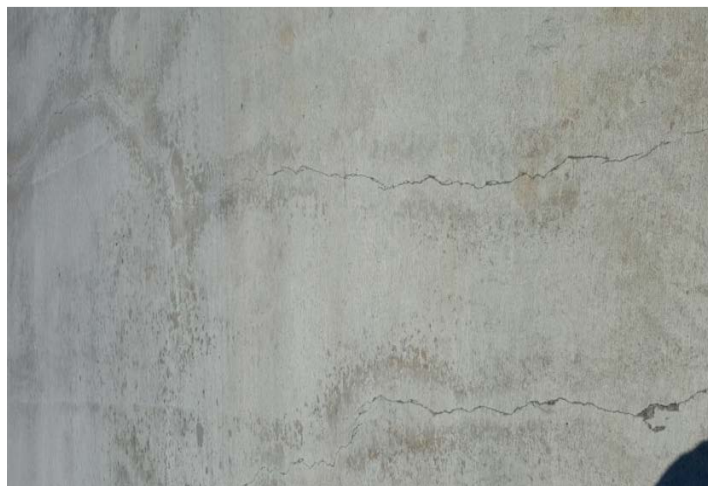
Figure 4. Control Slab Showing Cracking After 6 Months (the EdenCrete™ Slab Showed No Cracking After 6 Months)
