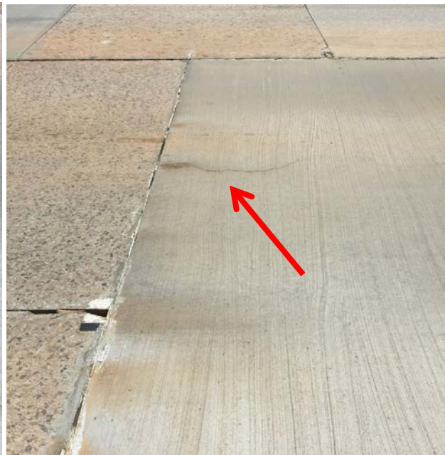
Figure 10. Control - Visible Crack Developing
