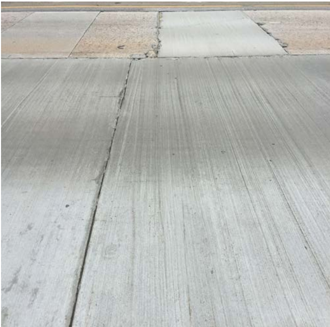
Figure 9. EdenCrete™ - No Visible Cracking
