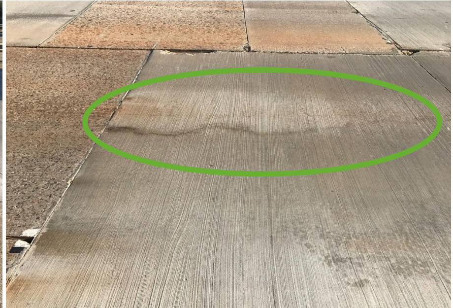
Control – Visible Crack Across Slab
