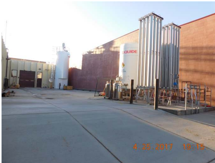
Figure 3. Liquid Nitrogen Storage tanks installed above underground bulk storage tanks.
