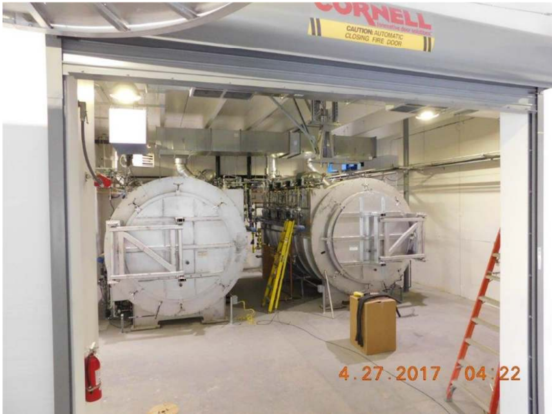
Figure 2. Reactors being prepared for final commissioning.
