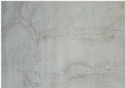
Control Trial Slab Significant cracks and wear after 6 months
