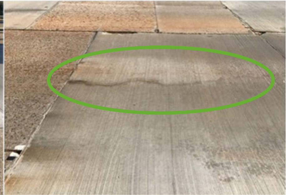
Control – Visible Crack Across Slab
