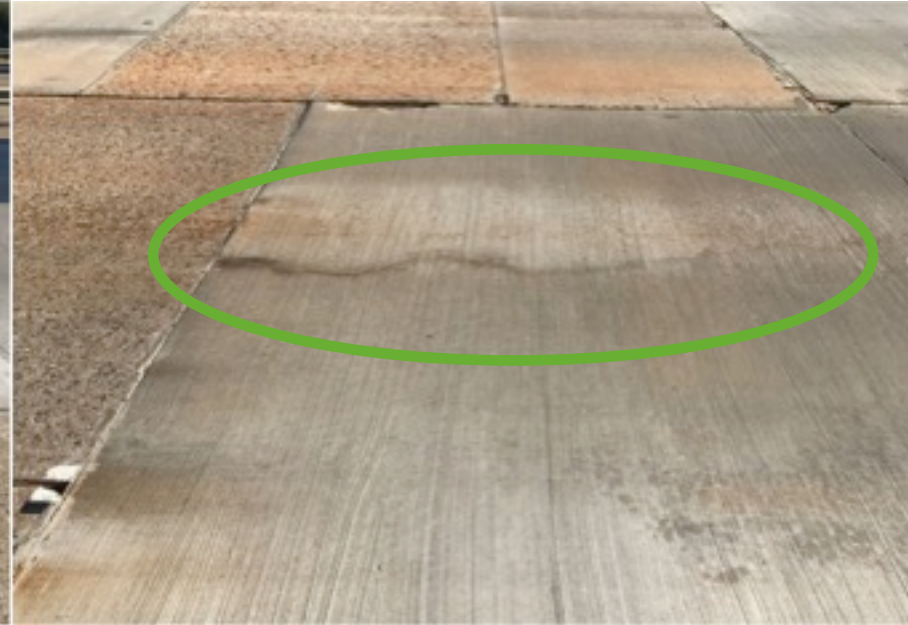
Control – Visible Crack Across Slab
