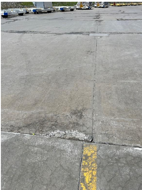
Figure 1. Section of worn concrete
