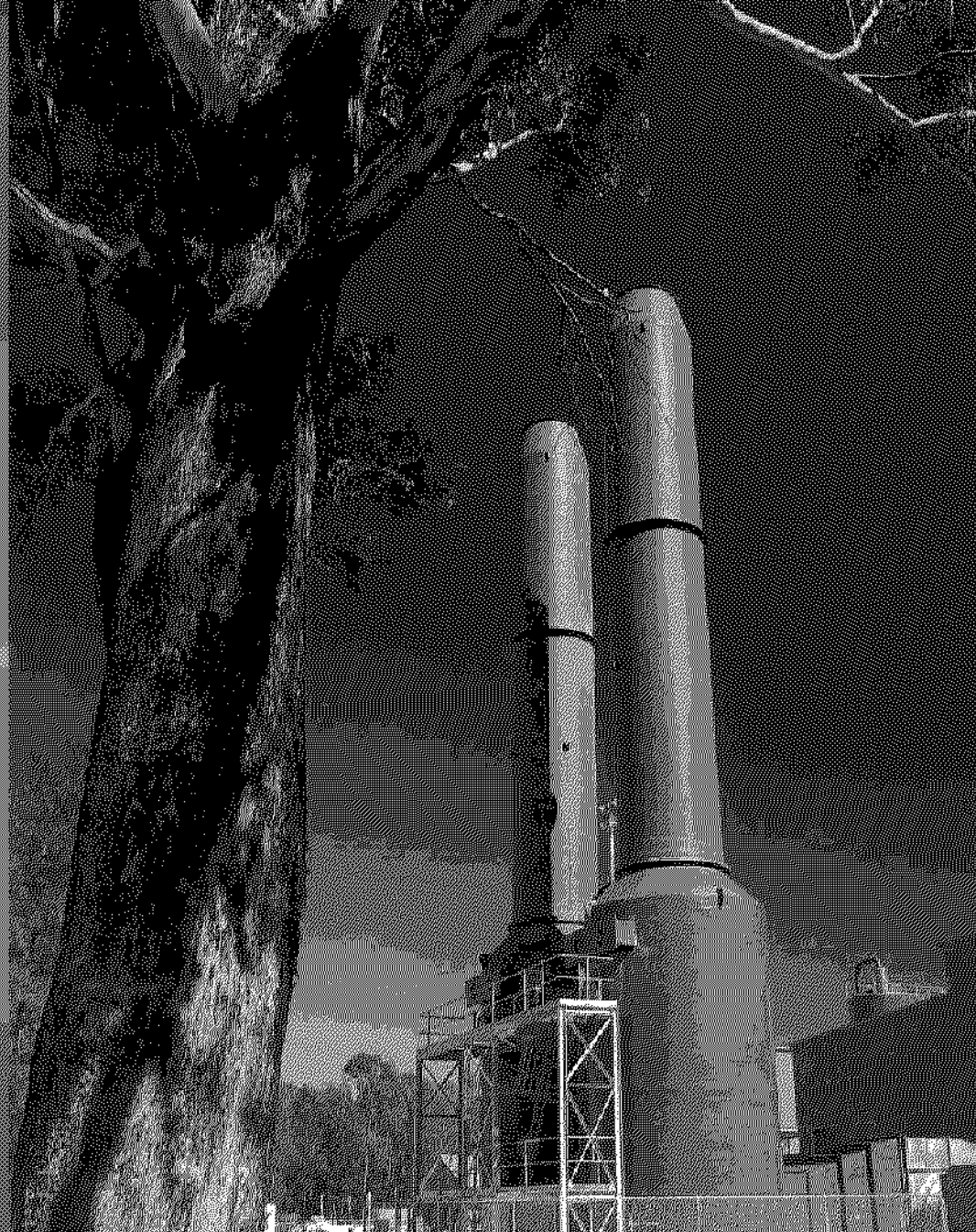
Odour Control System at St Marys Sewage Treatment Plant for Sydney Water.
